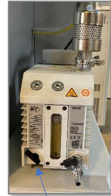
Vacuum Pump Ballast
